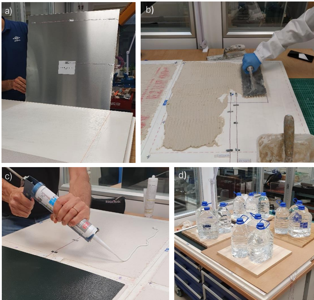
Figure 16. Pictures of the preparation of the (a) façade components, (b) the application of a mortar layer and (c) of the adhesive silicone for roof components, and (d) the drying phase, where weights were used to compress the panels.
