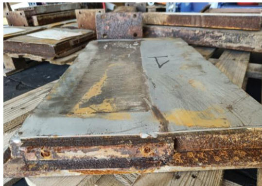
Figure 11 Deformation of the steel plate in multidirectional bearing
