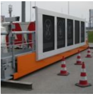
Figure 4: Installation of ultrasonic sensors on a gantry above the carriageway
