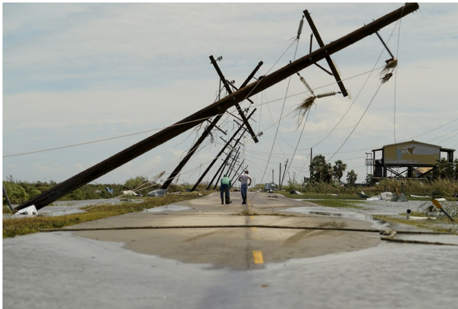
Figure 2-12 Downed power lines in Holly Beach, Louisiana, caused by Hurricane Laura on 27 August 2020 ( NBC News, 2020 ).
