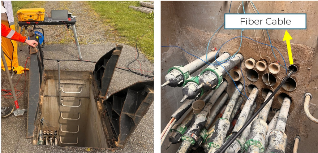
Fig. 4.11 Underground Technical Chamber
