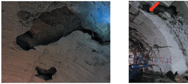
Figure 1. Examples of defects in tunnel lining with reduced thickness, identified during the refurbishment of the Monte Bianco Tunnel in Italy, after milling approximately 25–30 cm of the lining with a roadheader (courtesy of Traforo del Monte Bianco GEIE).
