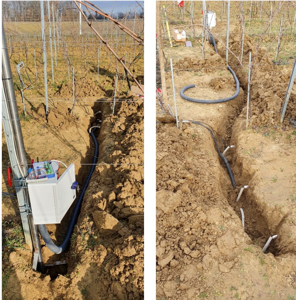
Figure 33: Installation at the vineyard in Capriata D'Orba of 12 probes for continuous soil monitoring (pole, solar panel, box containing battery and Siap-Micros microDA datalogger with 3G modem remotely connected for data transmission, probes for measuring soil water content Delta OHM HD3910.1 and related protective tubes for cables) carried out on 10/02/2022.
