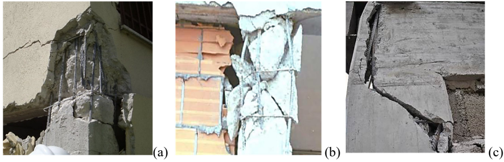
Figure 1.2: Example of damage due to structural deficiencies: (a) Poor detailing and design of the beam-column joints (Furtado et al., 2021); (b) Shear failure of column due to insufficient transverse reinforcement; (c) Shear failure of beam-column joint due to insufficient transverse reinforcement.
