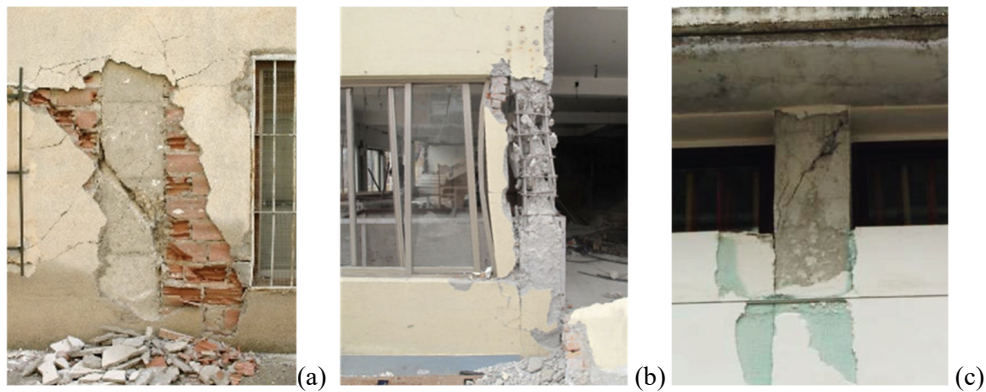
Figure 1.3: Example of short-column mechanisms (Sezen et al., 2000; Furtado et al., 2021): (a) Short column shear failure; (b) Short column double plastic hinge mechanism; (c) Short column shear failure due to openings.
