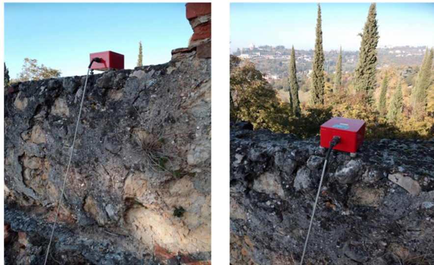
Figure 1. Example of a sensor installed on the top of the walls.
