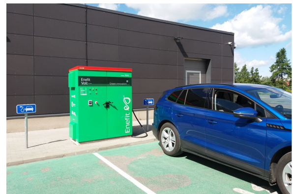
FIGURE 5. UC5 at Tallin's demonstration site: Superfast charging systems for EU corridors.
