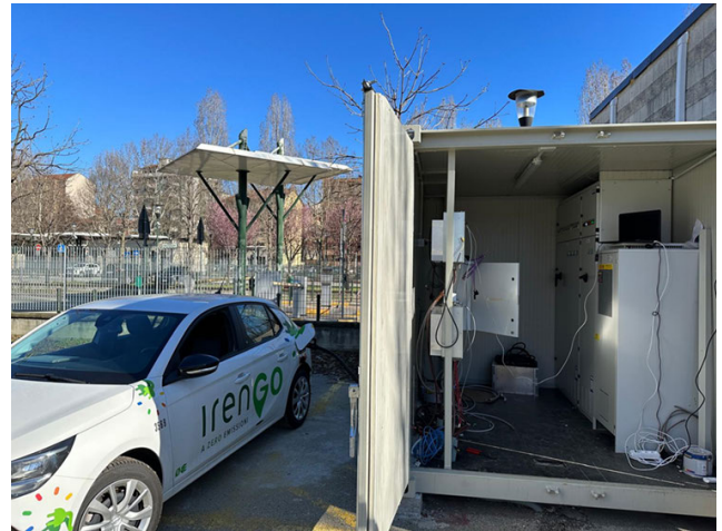
FIGURE 4. Charging session with detail of the container housing the cabinets and the 150kW power electronics.
