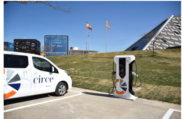
FIGURE 6. UC6 at Zaragoza's demonstration site:: Low power DC bidirectional charging infrastructure for EVs.
