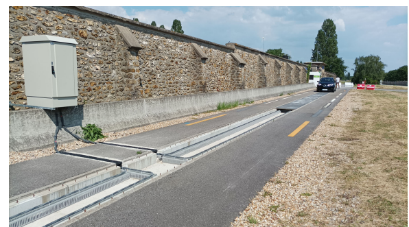
FIGURE 9. UC3 at Versailles demonstration site: partial view of the charging track and one of the supply cabinets.
