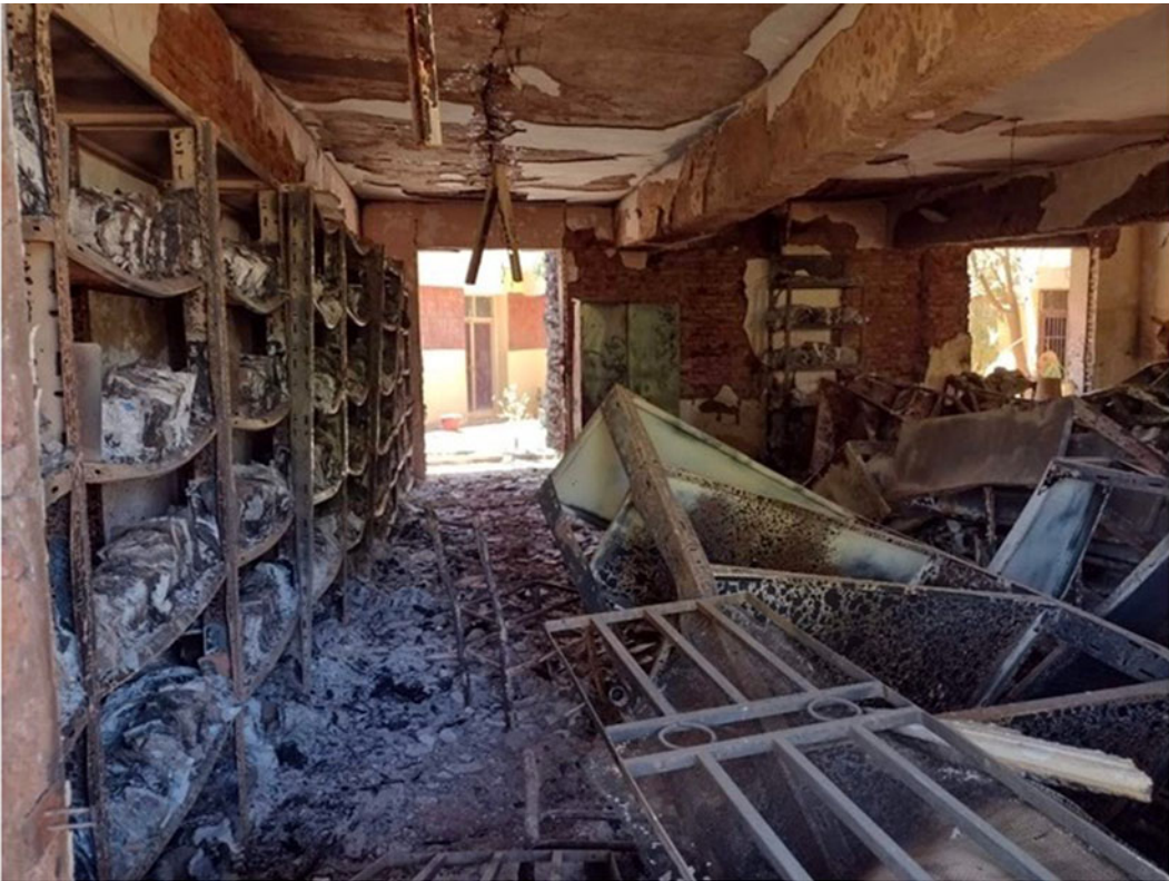
Figure 3. Documentation of complete destruction of Al-Omari Mosque, Jabalia, by direct shelling, as of November 7, 2023.
