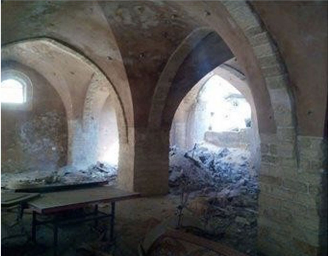
Figure 6. Documentation of damage to the Mohamed Omer Bashir Center at Omdruman Ahlia University.
