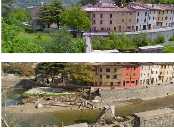
FIGURE 8. Pictures of the Cantiano bridge before (top) and after (bottom) the flood.
