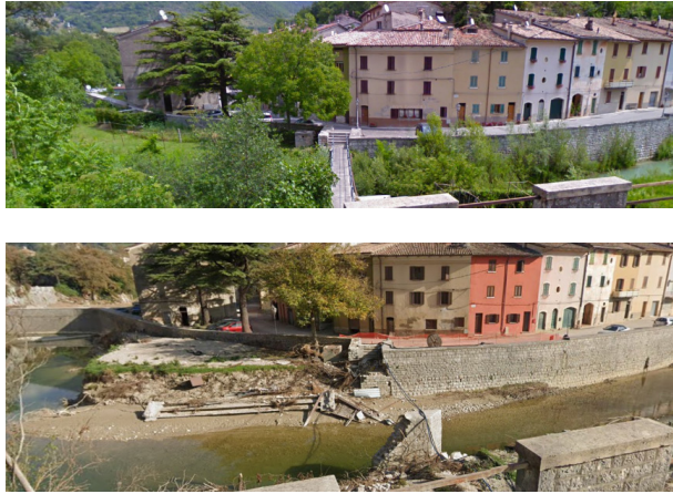
FIGURE 8. Pictures of the Cantiano bridge before (top) and after (bottom) the flood.
