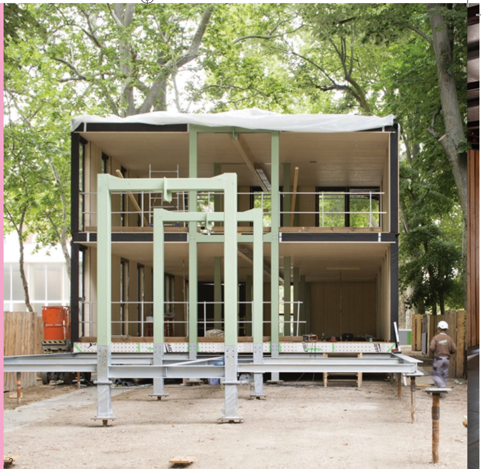
Fig. 2 Comparative composition. Left: Djuric & Tardio's itinérant crèche; right: Jean Prouvé's Croismare School (1948). The pairing underscores the kinship of portal-frame primaries and standardised envelope panels. Courtesy Djuric & Tardio Architects.
