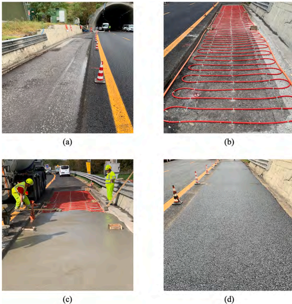
Fig. 14. a) Emergency lane after the milling operations, b) heat exchanger pipes arrangement and inspection manholes setup, c) concrete slab pouring and d) completely restored emergency lane.
