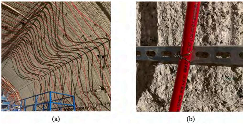
Fig. 7. Pipe pre-positioning through longitudinally wall-attached metal rods: a) view of the left springline and b) detail of the pipe-rod connection with metal wires.
