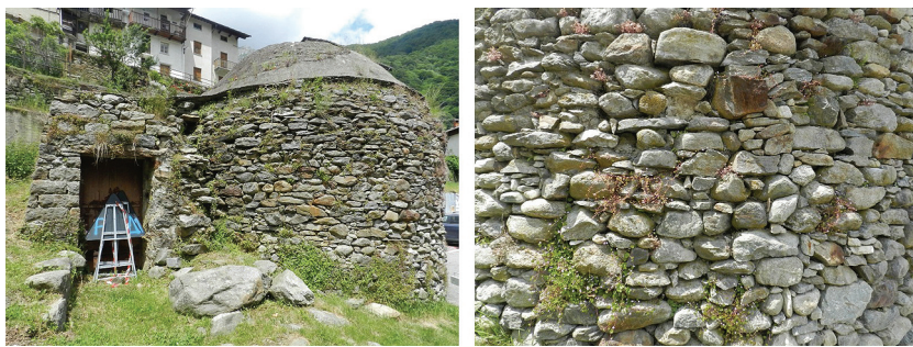
FIGURE 7 The Ice-House in Piedicavallo (left); A Detail of the Stone Masonry (right)
