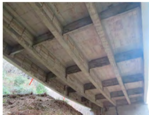
Figure 36. Viaduct case study 1—view of the girder layout of the RC ordinary reinforced concrete deck.
