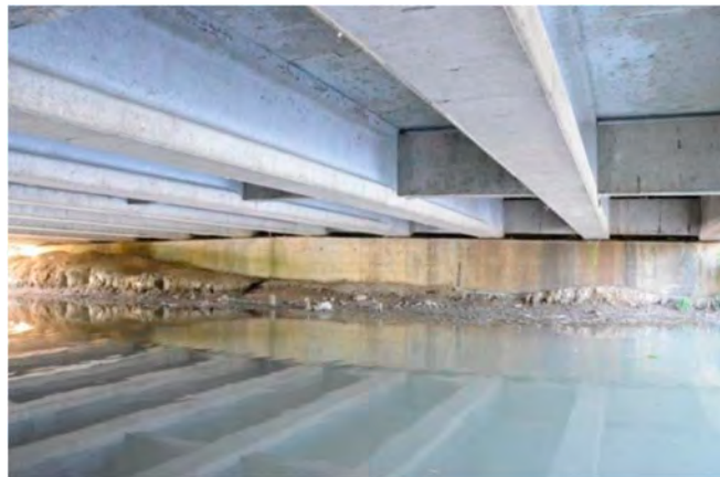
Figure 39. Viaduct case study 2—view of the girder layout of the PRC prestressed reinforced concrete deck.
