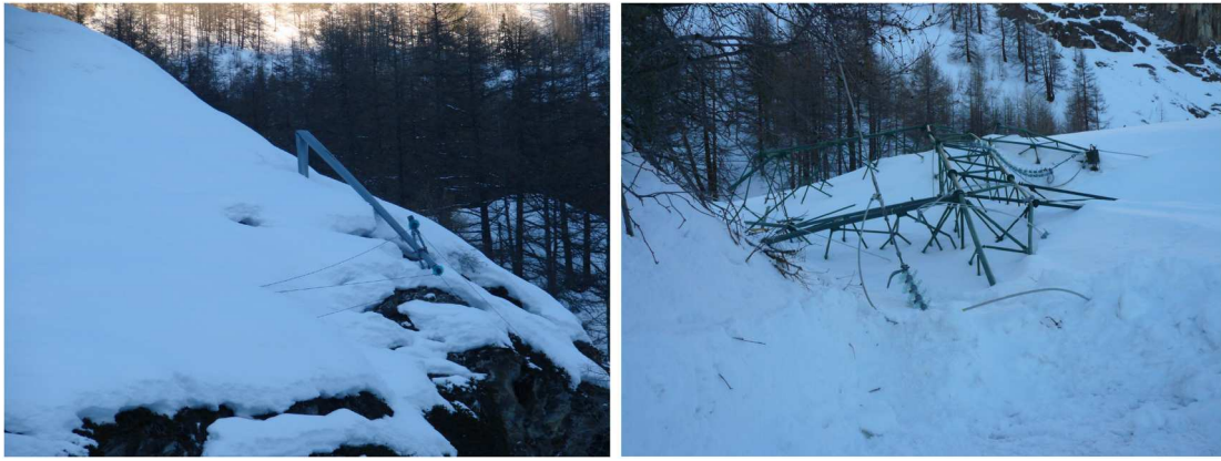
Figure 1. In (a), collapse of a steel pole due to the impact of a snow avalanche in Cogne, Aosta Valley, Italy, ref. snow avalanche no. V-12-121 on Dec 15, 2008. In (b), collapse of a power transmission tower due to the impact of a snow avalanche in Valsavarenche, Aosta Valley, Italy, ref. snow avalanche no. V-13-88 on Dec 8, 2018. The photos are publicly accessible at (RAVA, Ufficio Neve e Valanghe 2025).
