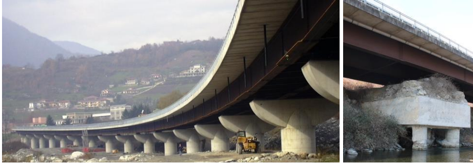
Figure 1: left, view of the Inverso Pinasca Bridge during construction (2004; Image courtesy of Seteco Ingegneria s.r.l.). Right view of current scouring conditions at pier P09 as of June 2023.
