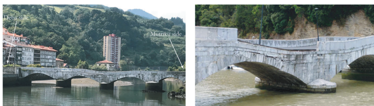
Figure 2. Deba bridge, Spain. The settlement of the central pier was induced by shipworm infestation in the timber foundation piles, from Malena et al. (2021).
