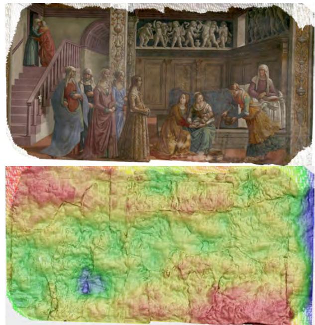
Figure 8. Santa Maria Novella Tornabuoni Chapel - west wall panel 2, Nativity of Mary. Visible layer above, slope and deviation map below.
