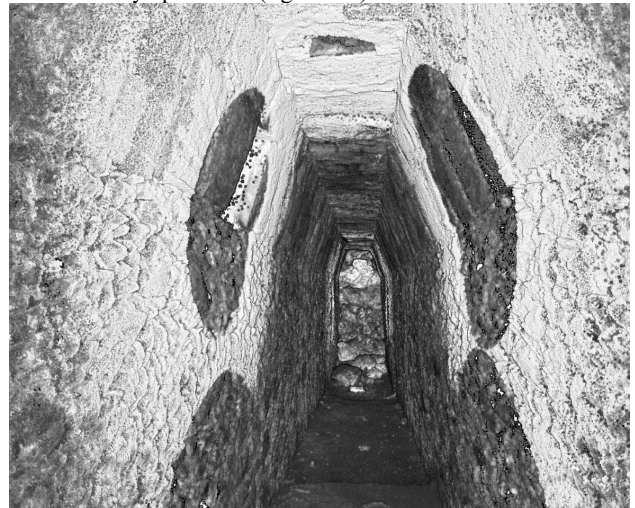
Figure 14. El Castillo South Tunnel interior, featuring distance-based deformations
