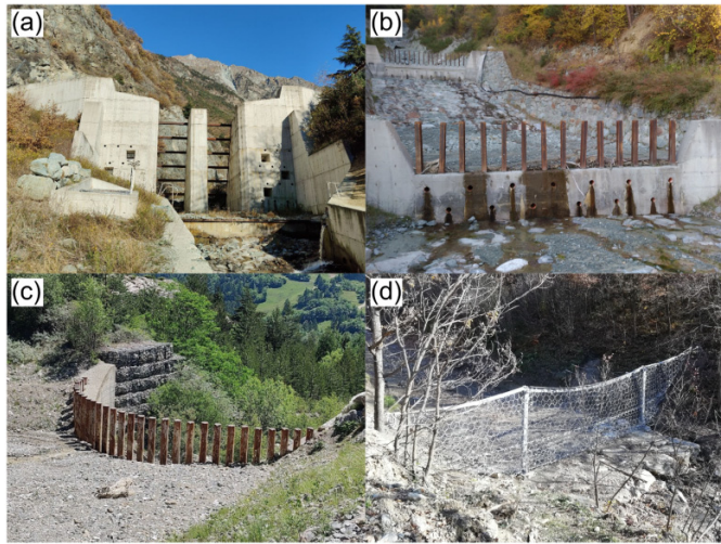
Fig. 1. Examples of typical barriers installed in areas prone to debris flows: (a) slit dam, (b, c) filter barriers, and (d) cable-net barrier.
