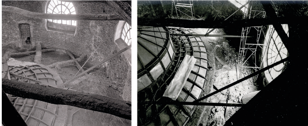
Fig. 4. State of conservation of the lantern before restoration works, c. 1984. Palazzo Carignano (Private archive of arch. Andrea Bruno).
