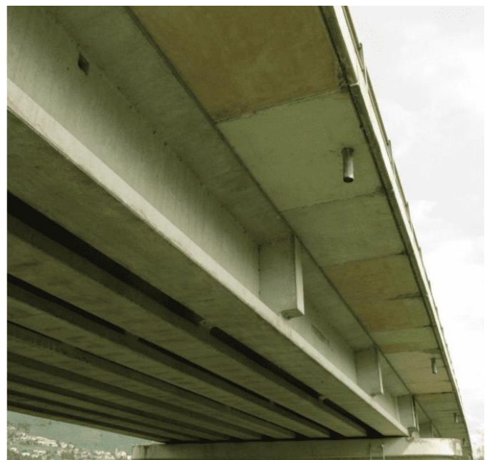
Figure 2: Intrados view of a typical span of the case study with the PRC beams.
