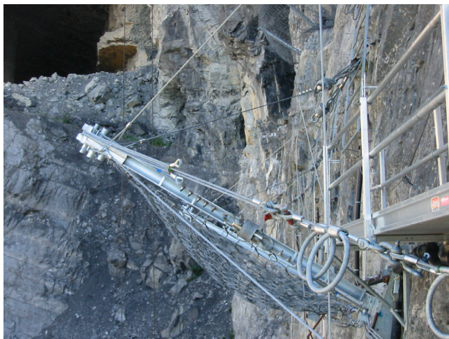
Fig. 12. Installation of the RXI-100 system during a full-scale test (image courtesy of Geobrugg AG).
