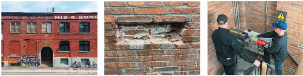
Figures 1, 2, 3. An existing building at 3558 Saint Patrick Street, Montreal, was selected as a case-study and used to collect detailed information on material and construction systems.
