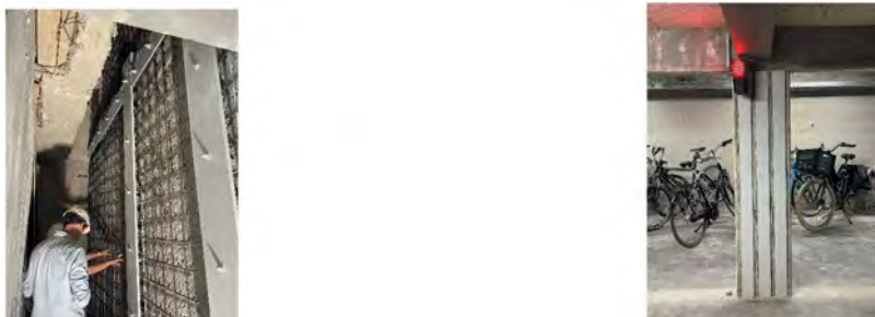
Figure 5. Left: The concrete core is reinforced by adding steel strips and profiles; Right: On lower floors, the needed glued-on steel strips seem almost-intentional decorative stripes. (©ono architectuur).
