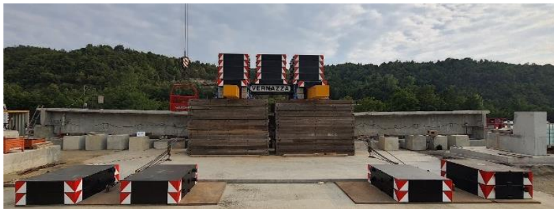
Fig. 7. View o of the PRC beam with around 50cm of deflection in midspan.
