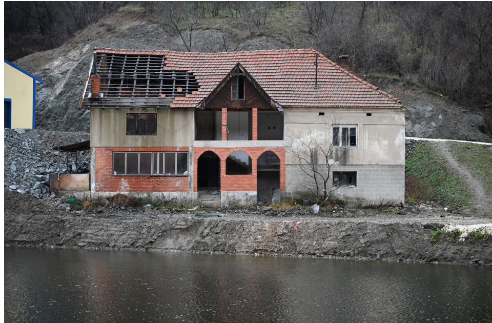
Figure 8. A photograph documenting a partially destroyed and subsequently demolished residential structure in Krivelj, Serbia, severely impacted by flooding caused by the rerouting of the Krivelj River in 2020. The flooding, a direct consequence of hydrological changes caused by mining operations, led to the abandonment of this home and its surrounding neighborhood. This area has since been designated as part of the Phase 3 flood control zone for the Veliki Krivelj open-pit mine, demonstrating the rapid transformation of residential land into operational mining infrastructure and highlighting the profound social and spatial disruptions experienced by residents. (Photograph by author, M.D., 7 December 2024.
