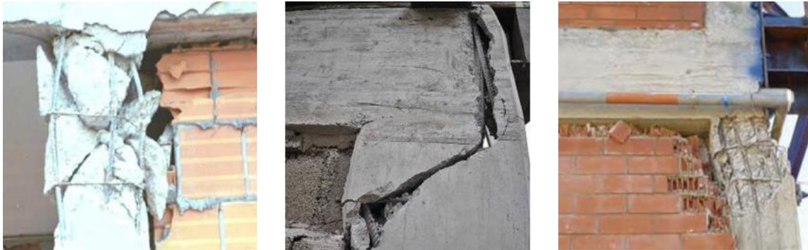
Figure 1: Local shear failure at column ends of infilled RC frames.
