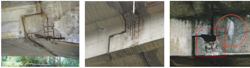
Fig. 1. Degradation of dapped-end beam bridges caused by steel reinforcement corrosion.
