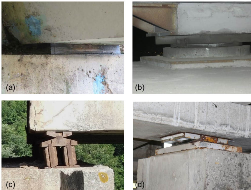
Figure 2. (a) Elastomeric, (b) pot, (c) steel, and (d) steel–Teflon bearings in inspected bridges.
