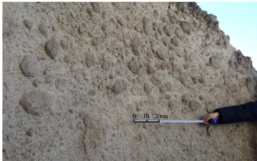
Fig. 3 A view from side wall of Koimesis Tes Panagias Church presenting various size of andesite blocks welding in a fine-grained matrix.
