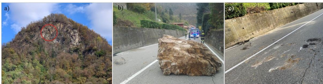
Fig. 2 a) detachment niche located on the Barbavara castle rock slope; b) kinzigite rock block of about 3 \text{ m}^3 that detached in November 2023, hitting the road; c) road damaged by the rock collapse.
