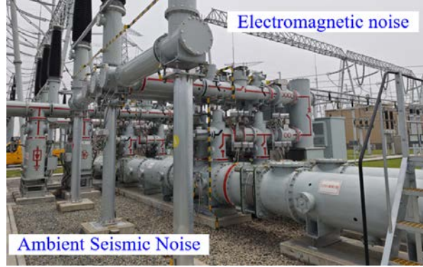
Figure 5-6 Noise sources in vibration-AE detection of GIS equipment
