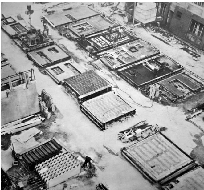
Fig. 4. View of the packaging and storage phases on the building site. Source: Gescal, IACP Turin, 1966.
