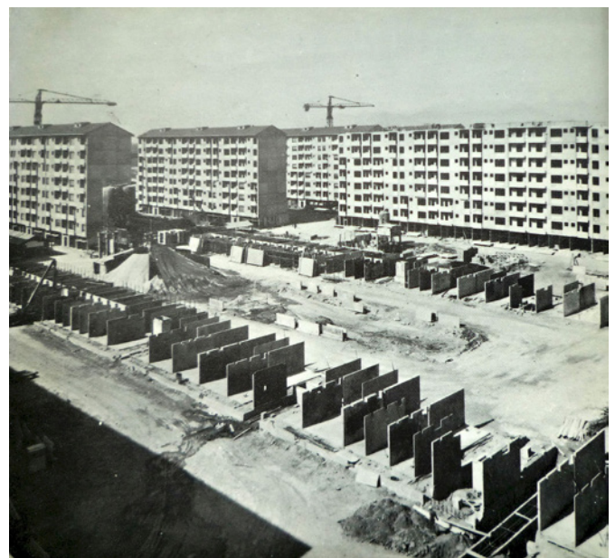
Fig. 5. View of the building site during the assembly phases of the load-bearing panels. Source: Gescal, IACP Turin, 1966.
