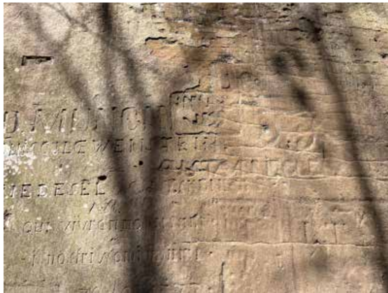
Figure 8. Area of the stone walls of the Fingalshöhle showcasing deterioration caused by weathering and water drainage.
