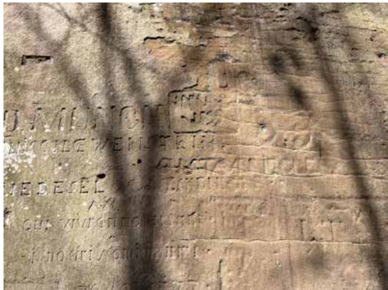
Figure 8. Area of the stone walls of the Fingalshöhle showcasing deterioration caused by weathering and water drainage.
