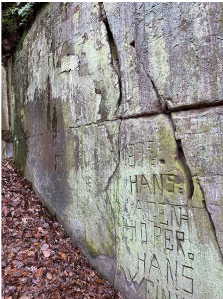
Figure 7. Area of the stone walls of the Fingalshöhle showcasing deterioration caused by weathering and the overgrowth with lichens, algae and moss.
