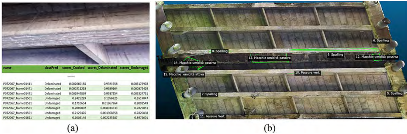
Fig. 9 (a) Example of an input image used for CNN analysis, along with the defect classification scores generated by the network. (b) Mesh model during the visual inspection process, showing isolated defects and areas of defect marked for defects of greater extent
