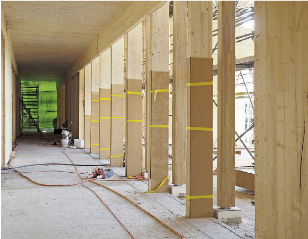
Fig. 3 | Construction site photograph of the central distribution corridor, showcasing the doubling of the vertical structure next to the double-height outdoor terrace (credit: Blumer Lehmann | Claude Hausammann, 2017).
