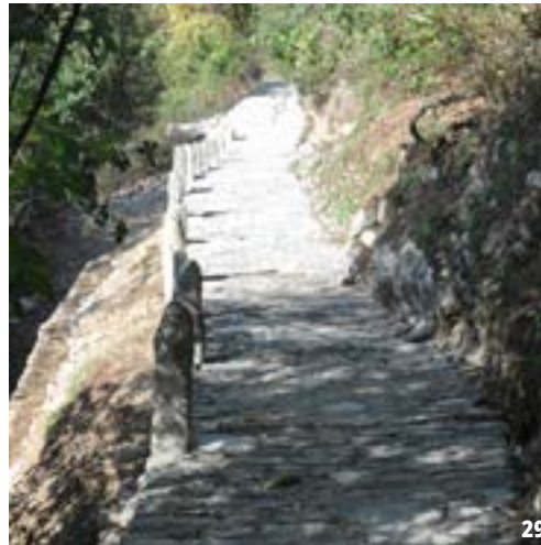
28-29. Before and after the kalderimi reconstruction, and the placement of the upright stones called arkades . Photo credit: G. Koutropoulos, P. Radin and G. Zoilis. Source: Boulouki Archive.
