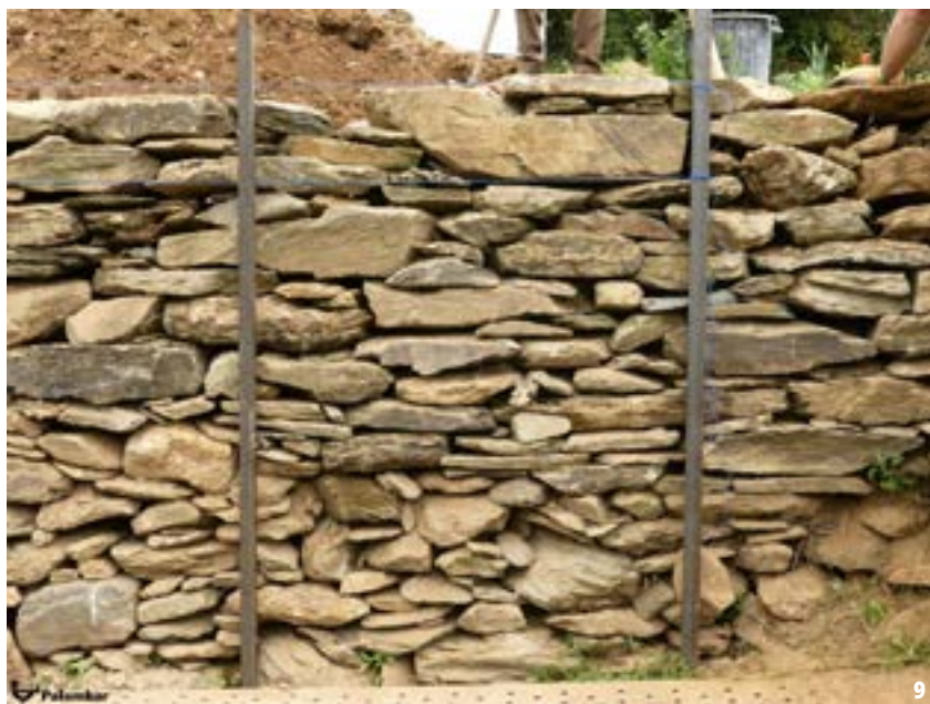
9. Construction of a dry stone wall during a workshop dedicated to the topic. Gaëlle Carvalho/Palombar 2019.
