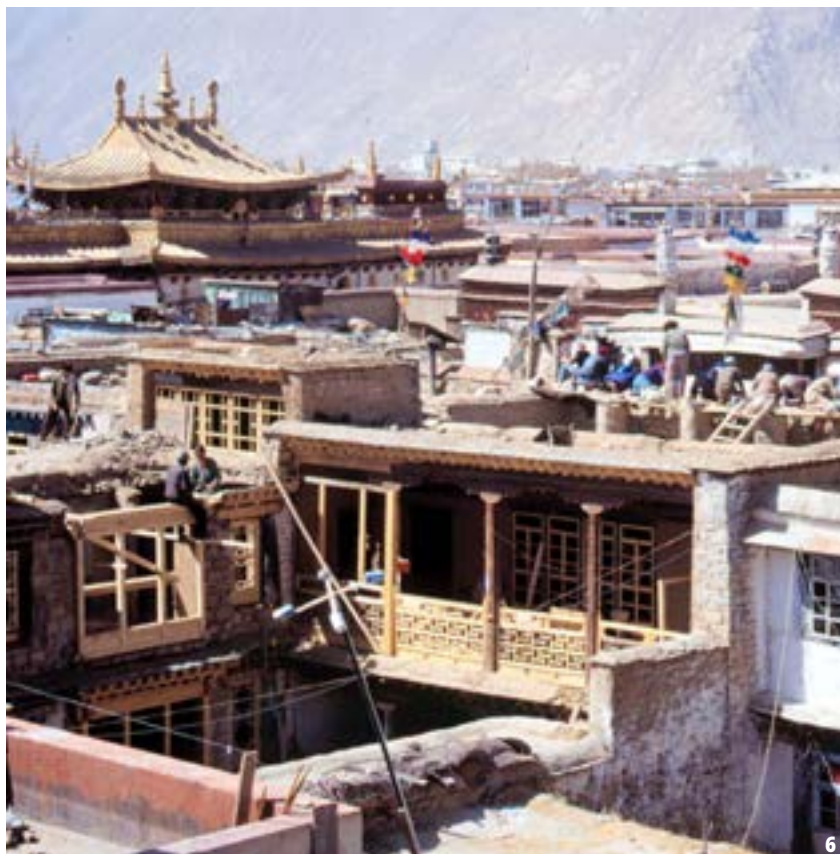
6. Restoration work of Rongdra House. Courtesy of Tibet Heritage Fund, André Alexander 1999.
