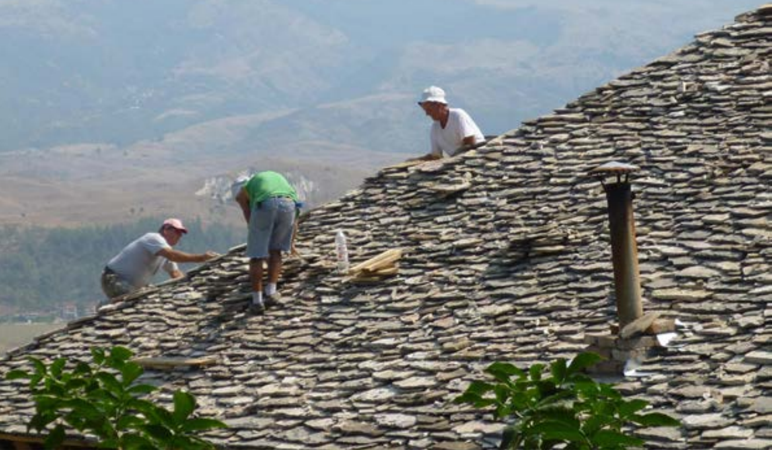
4. Stone roof restoration using traditional techniques in the frame of REVATO Project. Edvin Lamçe 2013.
