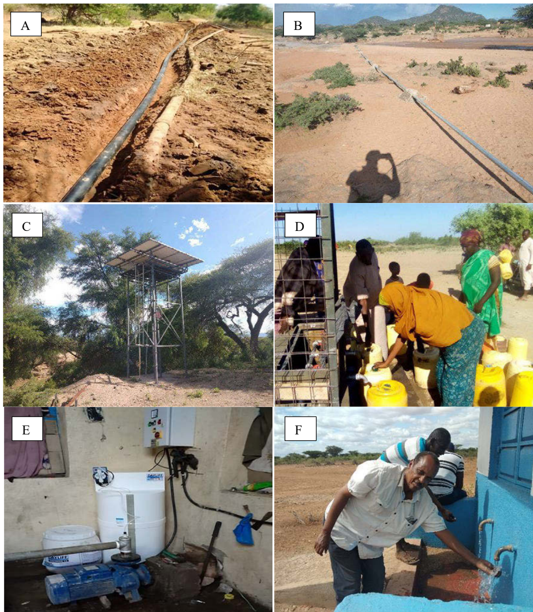
Figure 2. A) New installed HDPE pipes in the Bulesa village B) New pipeline in the Kipsing village. C) Borehole in the Kipsing Village with added solar panels for the new pumping system. D) Women fetching water at a community water point in Sericho village. E) Inline chlorine dosing equipment installed for Kinna village water supply system. F) The director of the water service during the launch of the new water kiosk in the Gafarsa village
