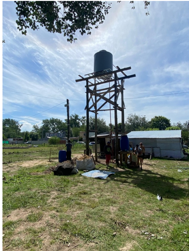
Figure 3 Water supply system. Image: Ana Vilenica
