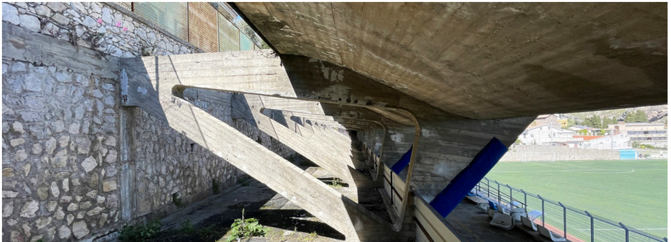
Fig. 3. The Nervi's skills emerges between fragility and degradation. Source: © 2021, Authors.
