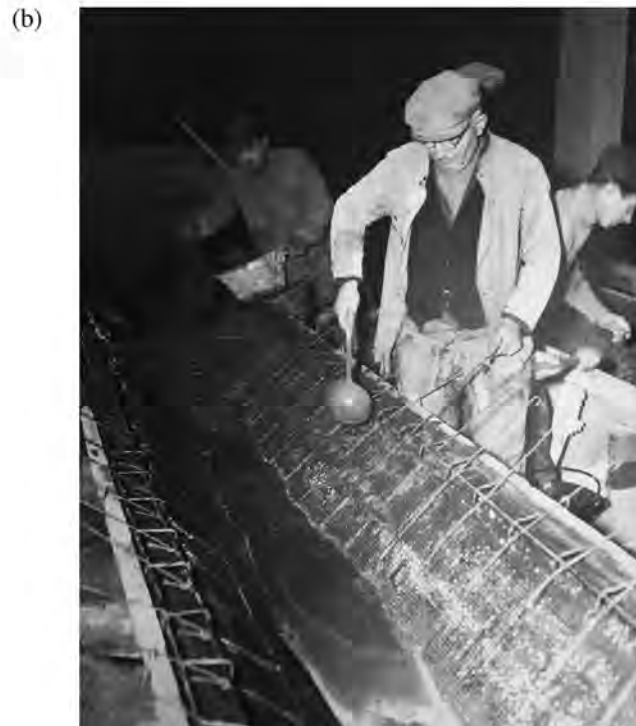
FIGURE 2 (a) Illustration of construction details related to ferrocement corrugated beams. 30 It is possible to appreciate the number of the wire mesh layers and the variations in thickness in the cross section. (b) Prefabrication on site of the undulated beams in ferrocement (1949–1950). 17
