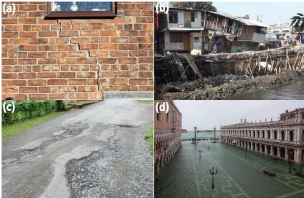
Figure 2.2: Examples of subsidence effects: (a) cracks in walls; (b) building damages in Jakarta, Indonesia; (c) road damage; (d) coastal flooding in Venice, Italy.
