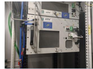
Figure 2 Installed electrolyser at ZEM module
