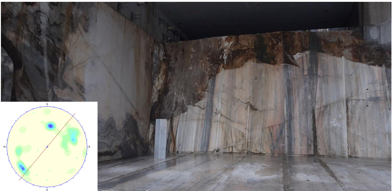
Figure 12. Bench opened in years 2020 – 2021, in the half-left side of the cavern, at the current level of the yard visible in the previous figure 3. Bench is about 5.5 m high. Joint with alteration is visible at face, lateral smooth cutting by wire saw is leaving an undisturbed surface and anisotropy of marble is put in evidence by alternate colors white – pink – grey or dark grey, following the main orientation of the subvertical vein and also of the embedding rocks. Stereonet of the joints in marble at the adit of the cavern is reported in the left corner: the red line represents the axis of the cavern.
