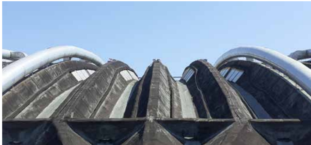
3c 5.6: A view of the impressive shape of the parabolic-like waves of Hall B, with surfaces not oriented in favor of the incidence of the projecting rays of the photogrammetric blocks of images.
