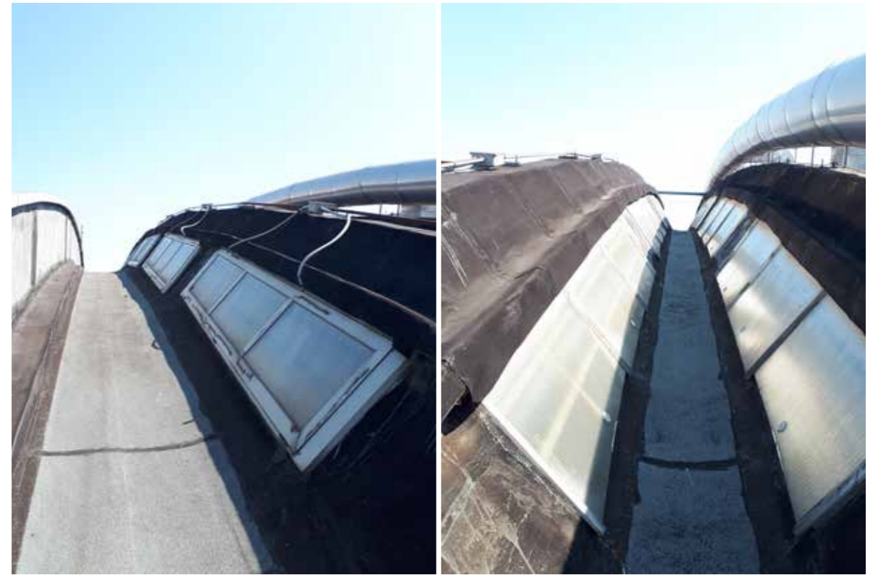
3c 5.8: Different types of skylights in the roof of Hall B, with an automatic opening mechanism that requires a larger frame and fixed openings
