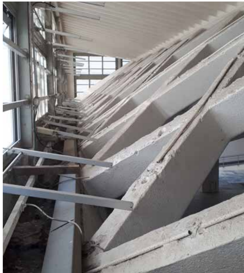
3c.5.2: A view of the vaulted portion of Hall C without panels between the ribs to allow the hall to be illuminated.
