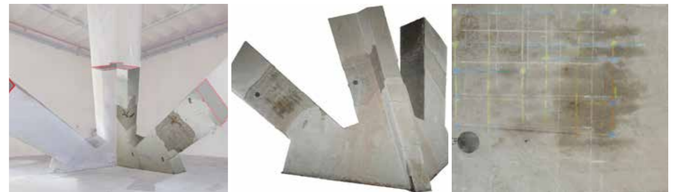
3a 9.5: Texturized model of the base of the arches, enabling corings, cracks and exposed iron to be located, and the positions of the sensors used during diagnostic investigations. Below: an example of orthophoto of a recognition area of the column reinforcement grid.
